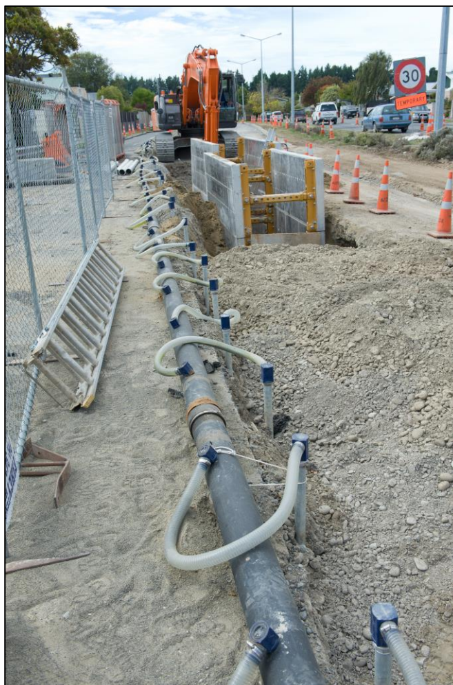
Pipe away: Water is removed from a work site in Christchurch's East.
