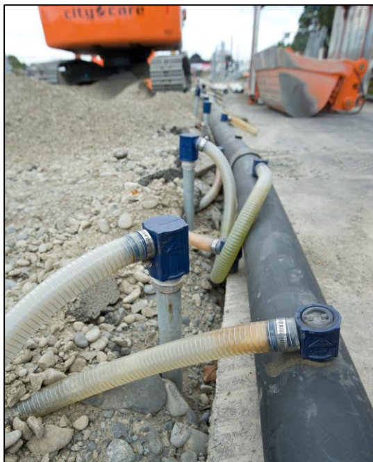
Soggy situation: Water is removed from a site so excavation can begin.
