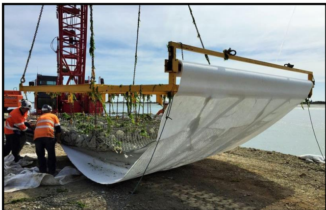
Putting it to seabed: SCIRT workers prepare to lay the Reno mattress on the sea floor.
