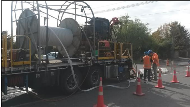
All wound up: The Spiral Wound pipe lining technique in use in the suburb of Fendalton.
