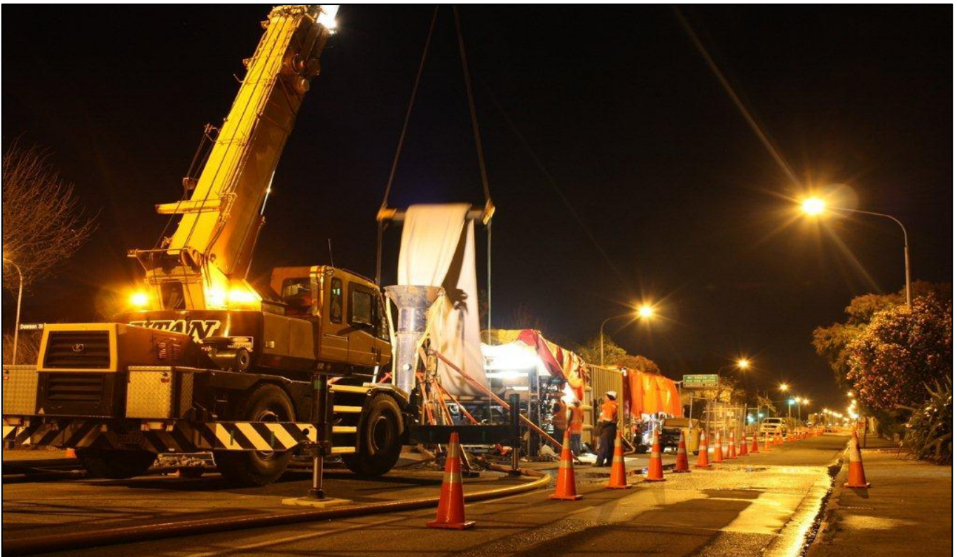
Cool approach: Large diameter CIPP lining took place in the cool of night to prevent the resin from curing in Kilmore Street, central Christchurch.
