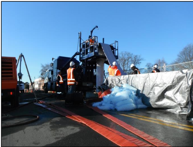
Line up: A SCIRT team uses Cured-in-Place-Pipe lining in the central city in Christchurch.
