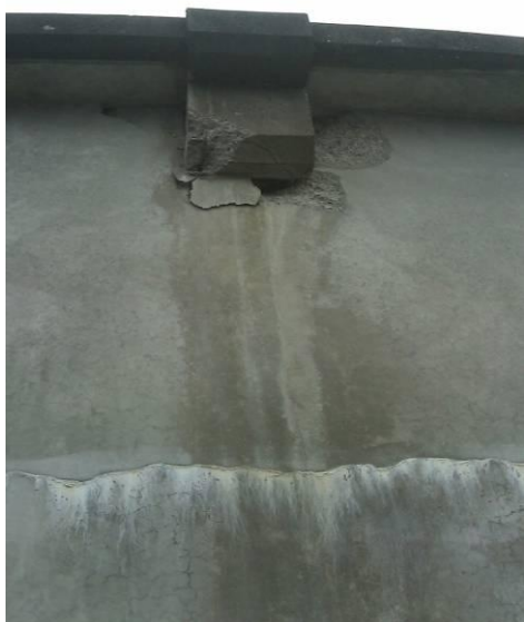
Figure 10: Upper Balmoral Reservoir – concrete damage at roof beam wall support.
