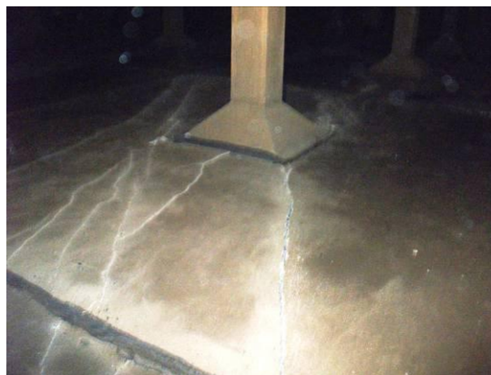
Figure 2: Huntsbury No.1 Reservoir – base-slab cracking.
