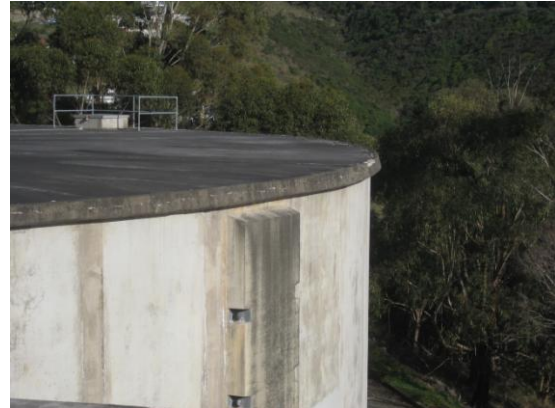
Figure 4: McCormacks Bay No.1 Reservoir – significant roof damage.
