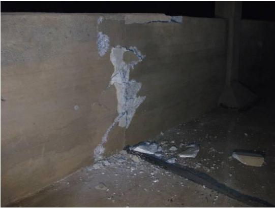
Figure 3: Huntsbury No.1 Reservoir – dividing wall failure.
