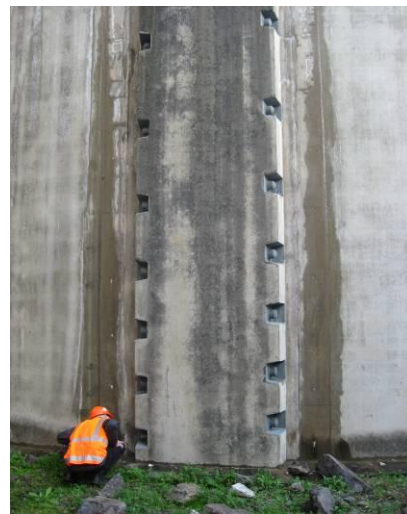
Figure 5: McCormacks Bay No.1 Reservoir – leaking vertical construction joints.
