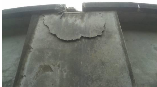
Figure 9: Upper Balmoral Reservoir –concrete shear failure at pilaster locations due to roof beam (concealed) impact.
