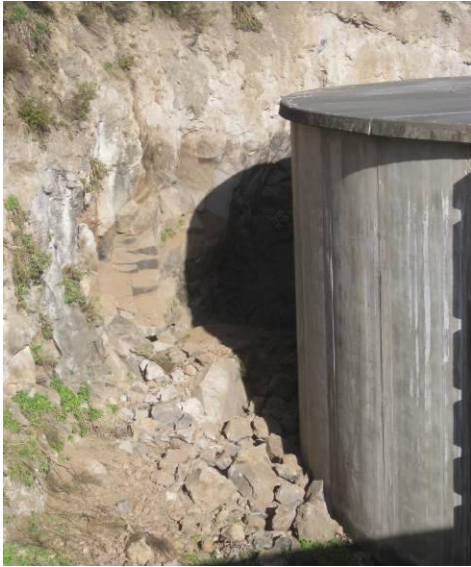
Figure 6: McCormacks Bay No.1 Reservoir – rock fall behind reservoir.
