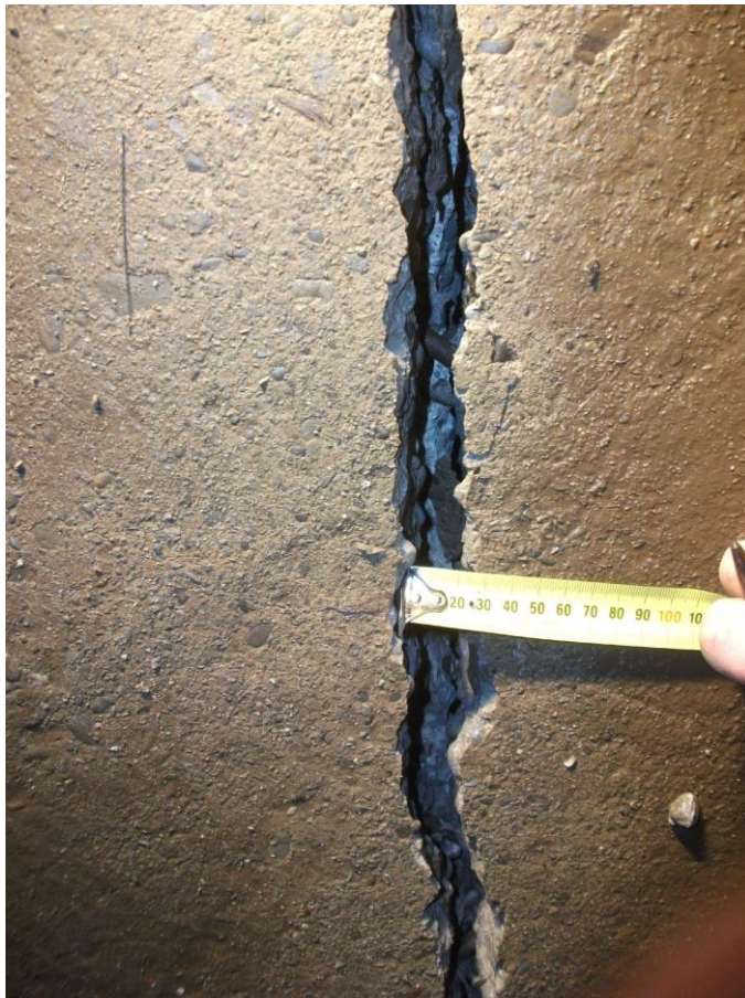
Figure 4: Crack in Floor Slab
