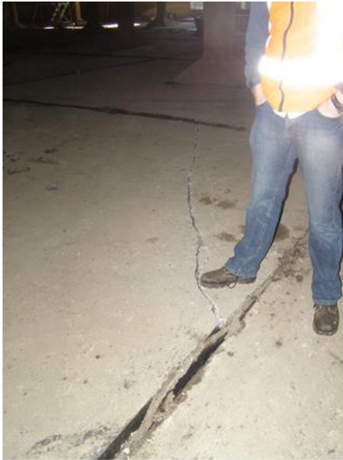
Figure 3: Dislocated Floor Slab Joint
