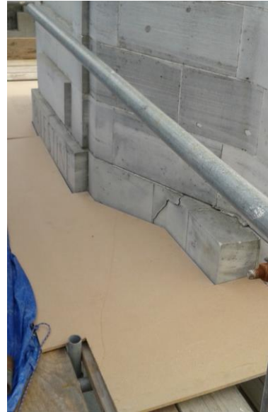
Visible Cracking in South Major Column
