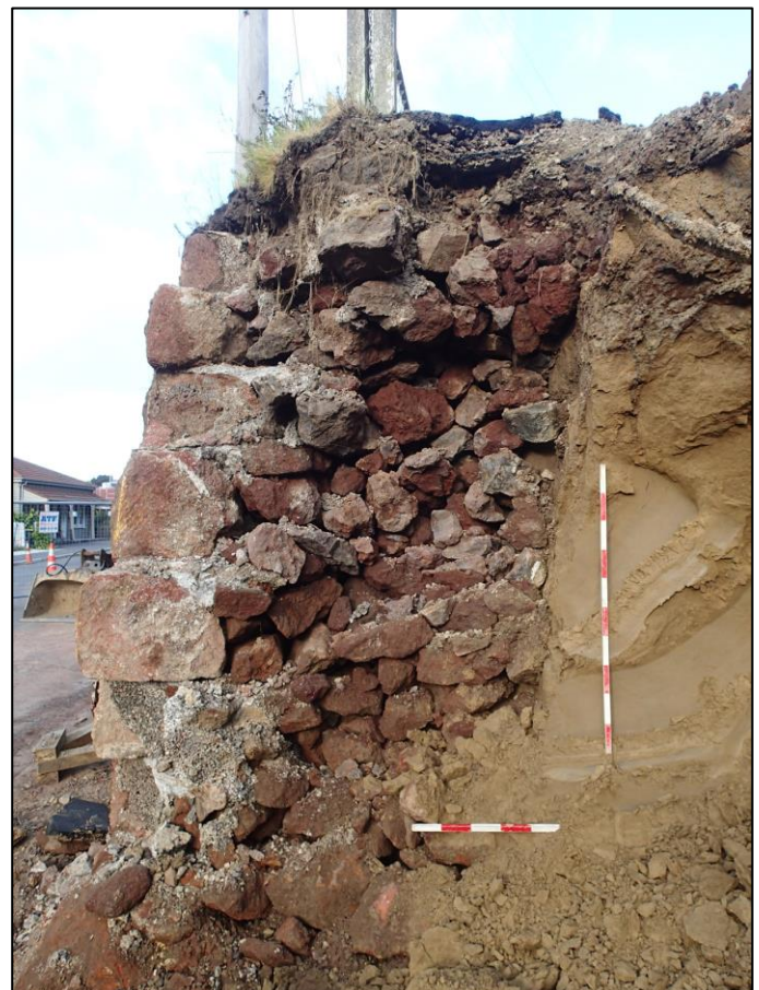
Another brick in the wall: A “red rock” retaining wall in Lyttelton reveals several crumbling layers.
