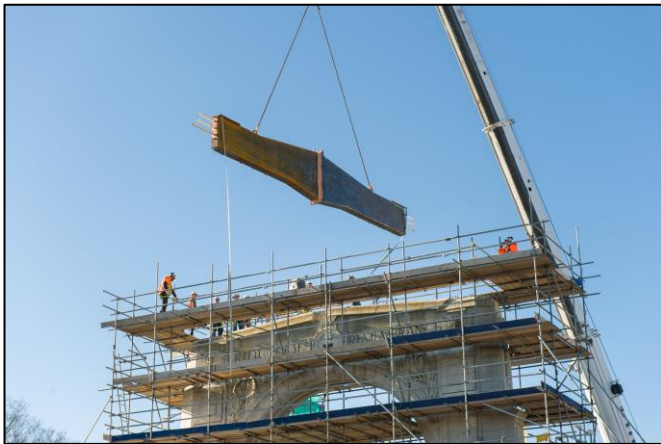
An 8.2-tonne beam with a central sliding plate is hoisted into place on the Memorial Arch.
