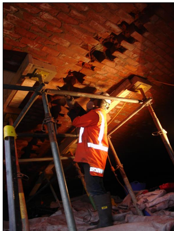
Brick up: A worker fills the gaps under the Armagh Street Bridge
