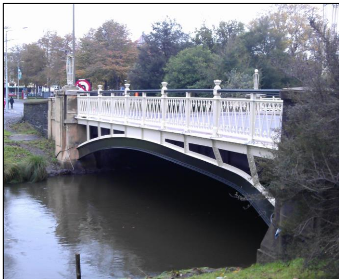
Side warp: A warped girder on the Colombo Street Bridge.
